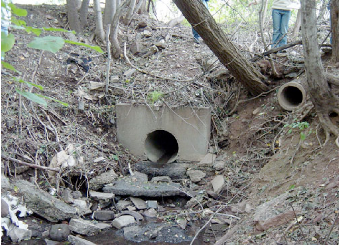
Figure 4a: Six storm drains empty urban runoff directly into the Teaneck Creek.
