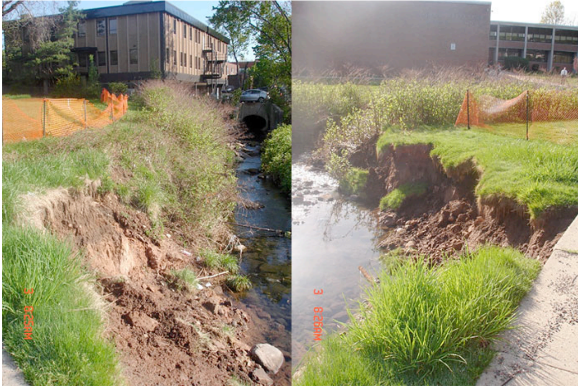
Figure 4: Erosion downstream from discharge pipe at Thomas Jefferson Middle School.
